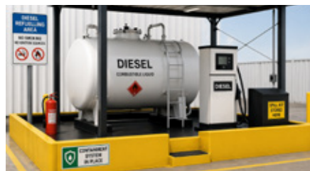
Secondary containment systems installed in diesel refuelling areas
